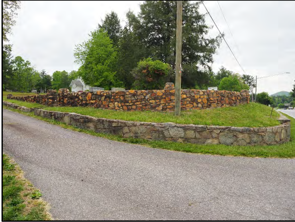
Figure 29: Cut stone embankment wall beneath the river rock walls and along the entrance drive, looking northwest.
