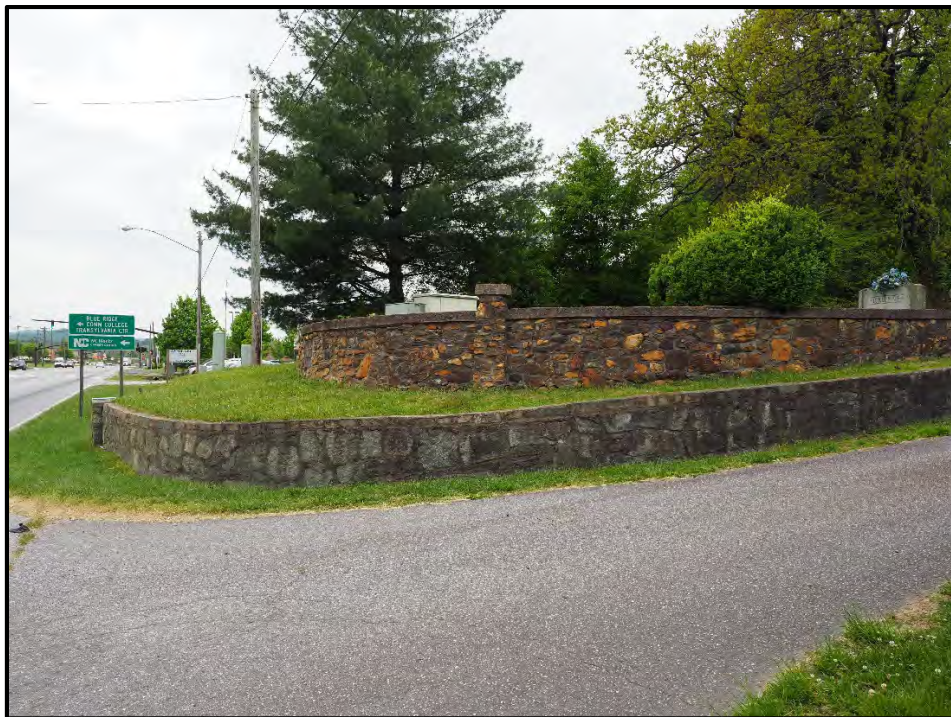
Figure 30: Cut stone embankment wall beneath the river rock walls and along the entrance drive, looking south.
